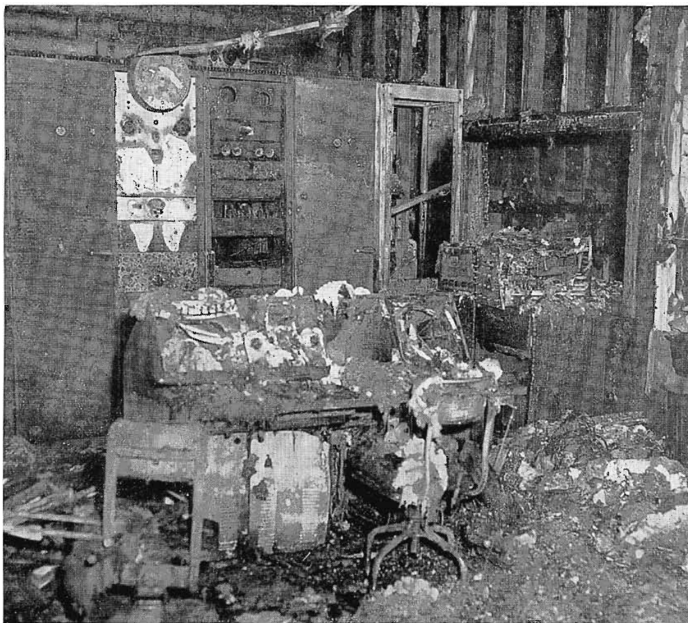
Fire damage in the WCOV-TV studio. One of many scenes of devastation throughout the building. Station back on air in twenty days with new RCA equipment.
