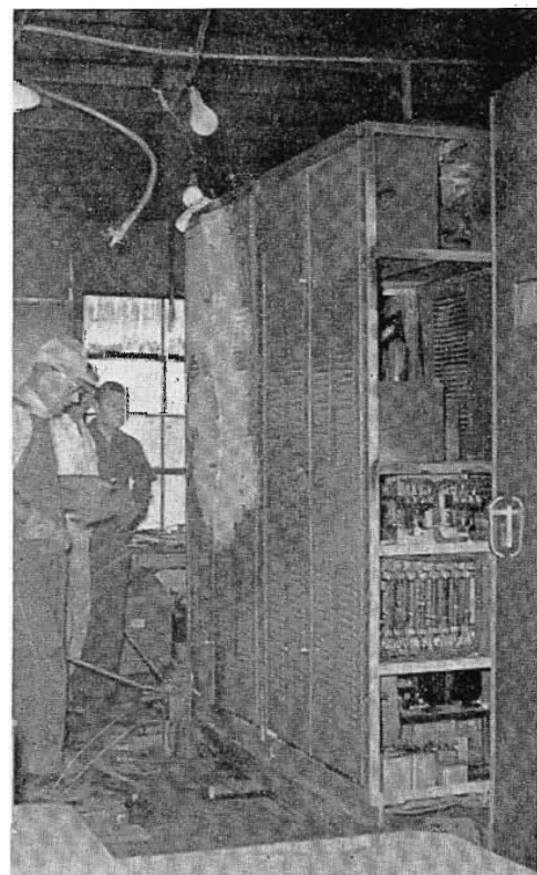
WHBL fire damage in transmitter building. Adjacent RCA FM transmitter, shut off during fire-fighting, returned to air in less than one hour.
